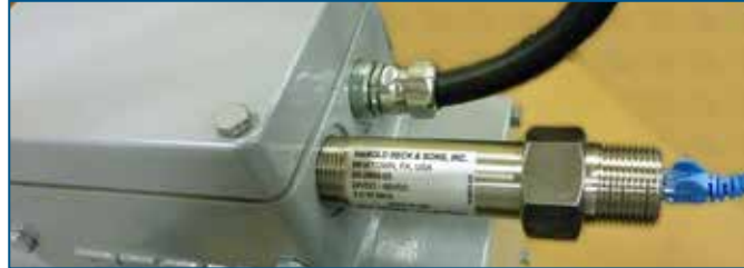
INSTALLED BECK MODBUS TCP ADAPTER
