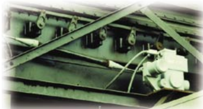
Beck drive installed on utility boiler lower damper
