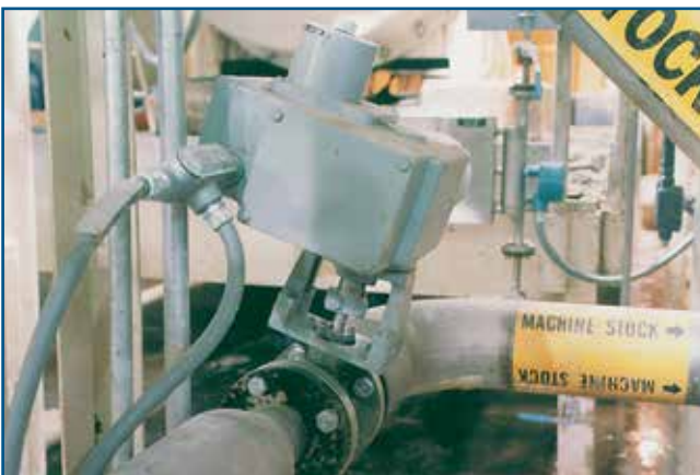
Machine chest level control valve
