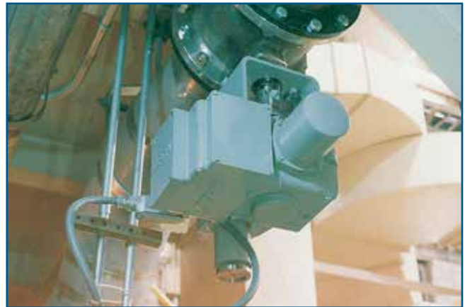
Stuffbox level control valve
