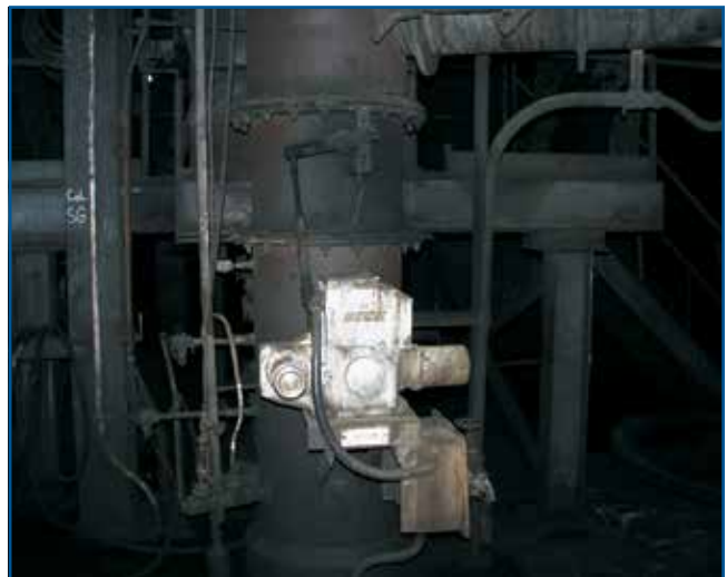
Beck actuator installed on a coal mill exhaust damper.
