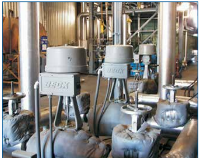
Group 14 linear actuators on condensate return valves.
